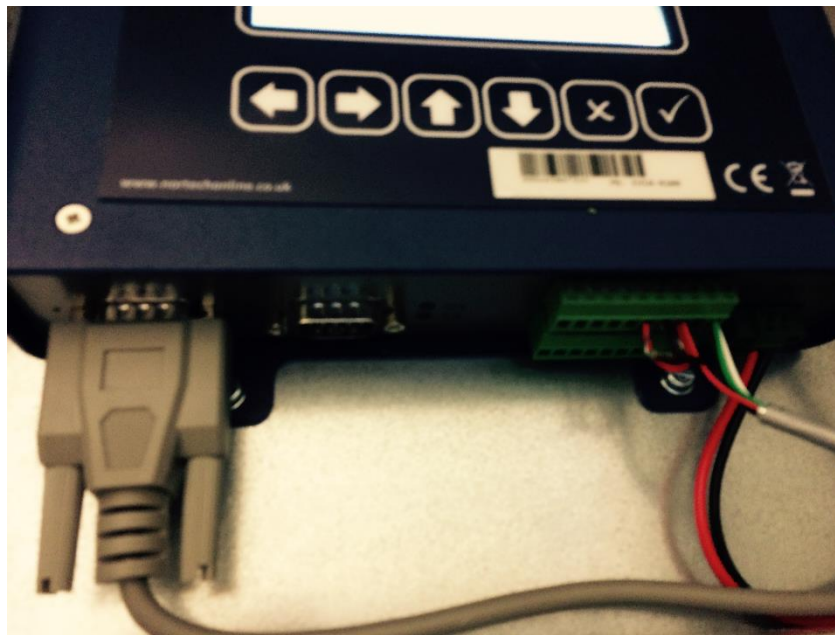
Figure 3. Nortech EV10 with MODBUS RS485 port (green).
