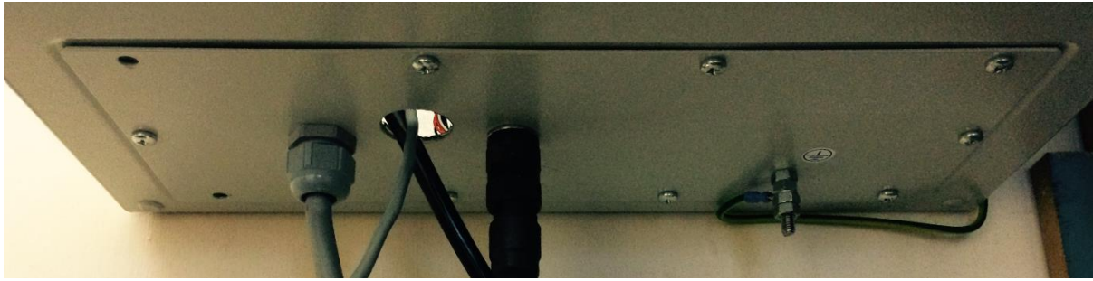
Figure 2. MC Enclosure bottom plate with Rail 350v MODBUS and power supply cable. Note, gland not shown. Note Class 2 enclosure on Lyndhurst site will be a polymer class II.
